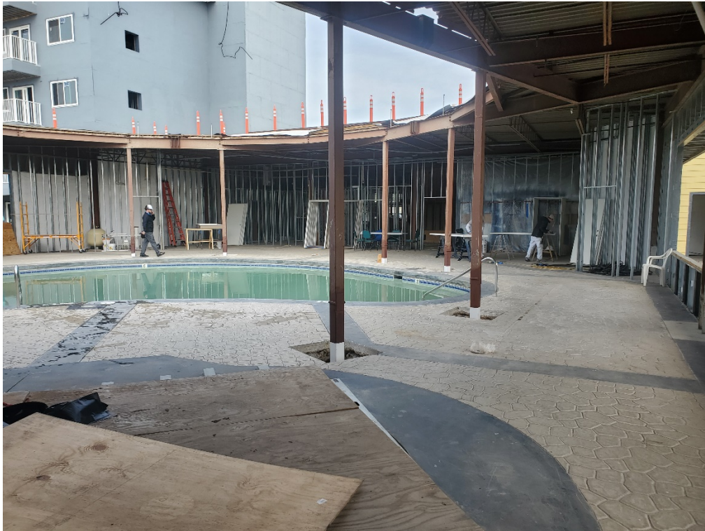
MAIN COLUMNS HAVE BEEN REPAIRED AND EPOXY COATED FOR BELOW GRADE PROTECTION
